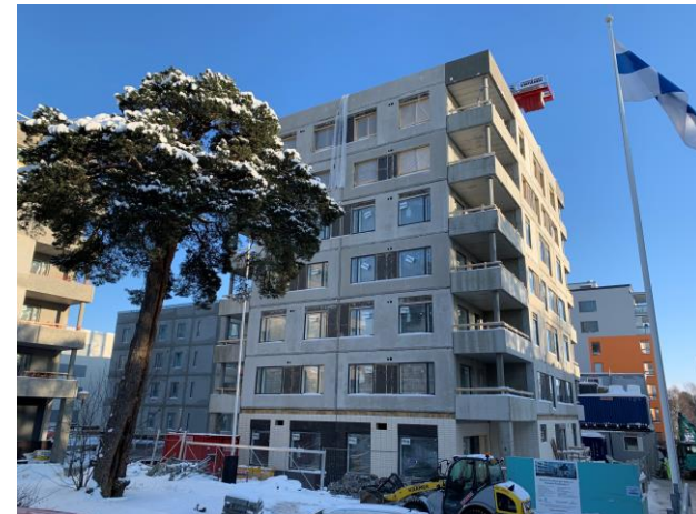
Photo from the eQ Residential fund site in Laajasalo in Helsinki on February 5, 2021. Asunto Oy Helsingin Kaiku 4 / Yliskylän Puistokatu 7, 43 apartments. The site will be completed in December 2021.
